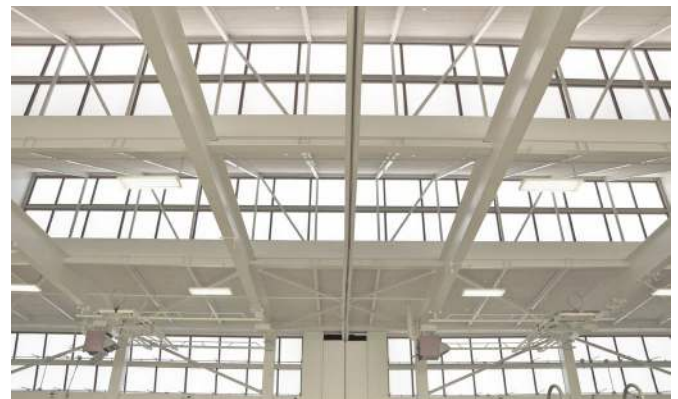
TechVent 5300 windows at MLK elementary in Berkeley, CA
